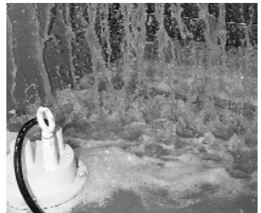
Filtered water collects in water tank for discharge into sewerage or recirculation system.
